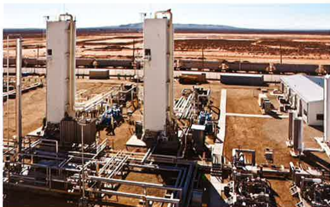
FIG. 9. An LNG plant with multiple trains. Photo courtesy of Clean Energy Fuels.
